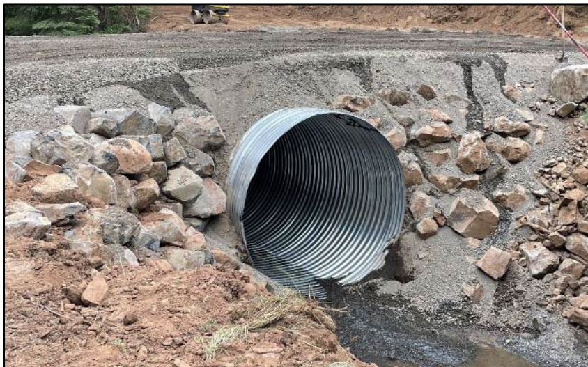
Figure 9-1) Example of a newly installed culvert on Tribal forestlands.
